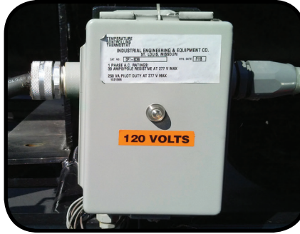
Over night heating system.
